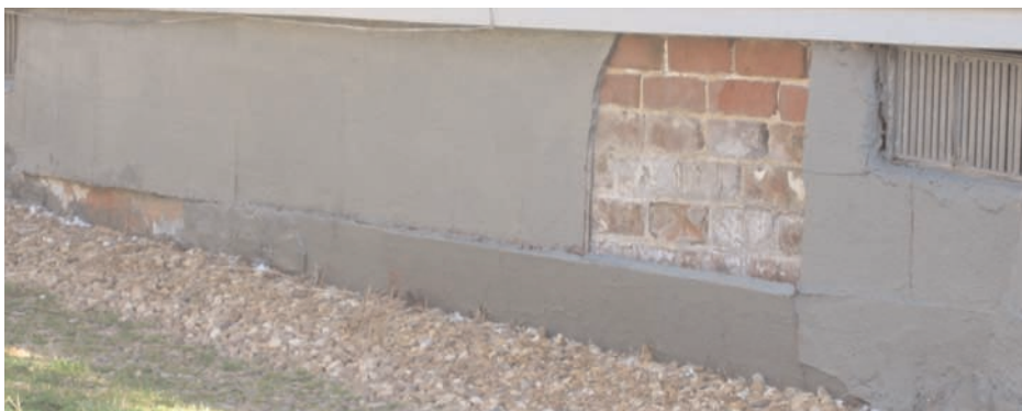
Moisture problems can cause paint failure on masonry (top) and block the adhesion of secondary coatings such as the parging seen here.
