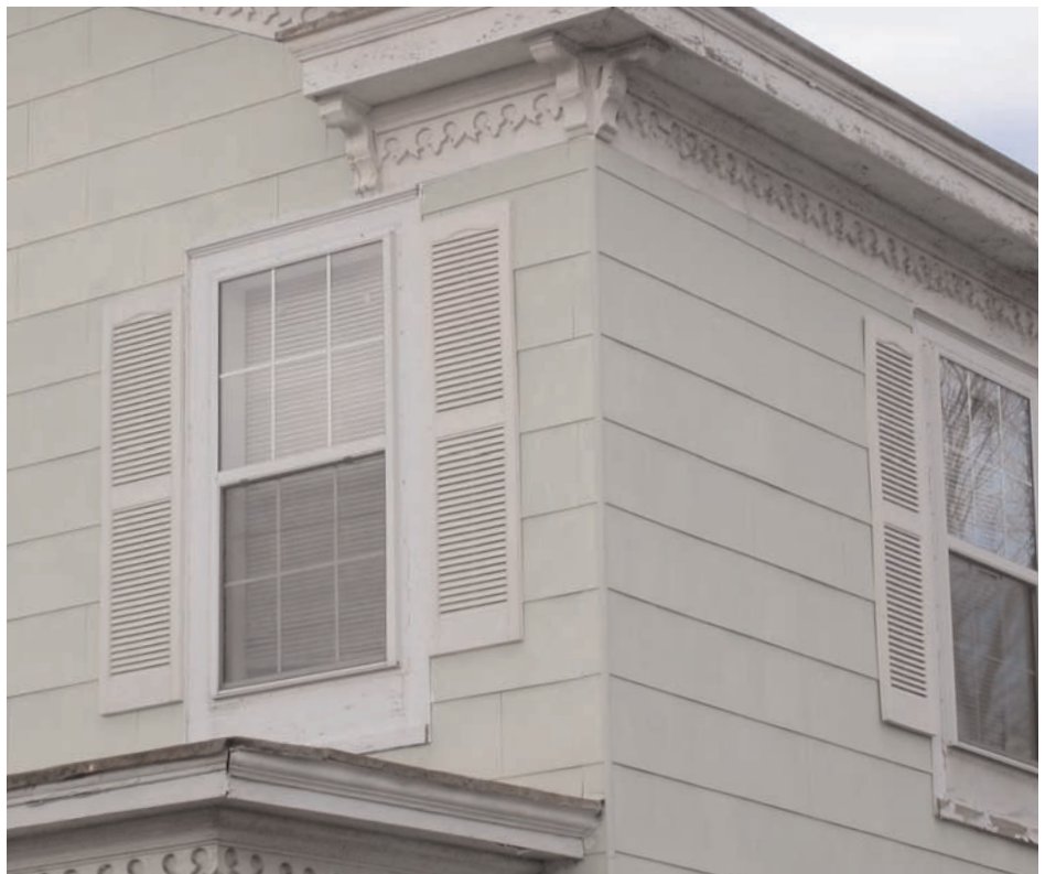
Replacement windows do not fit existing opening.
